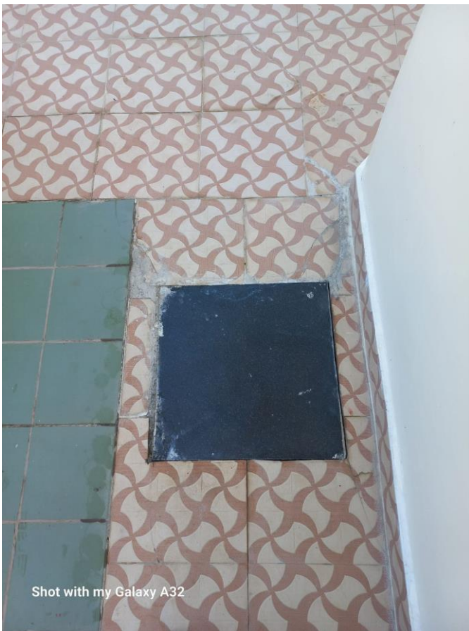
Fig -3: Drain chamber (black) and the broken tiles (refitted)
